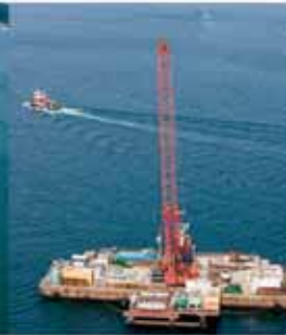
Offshore water intake
